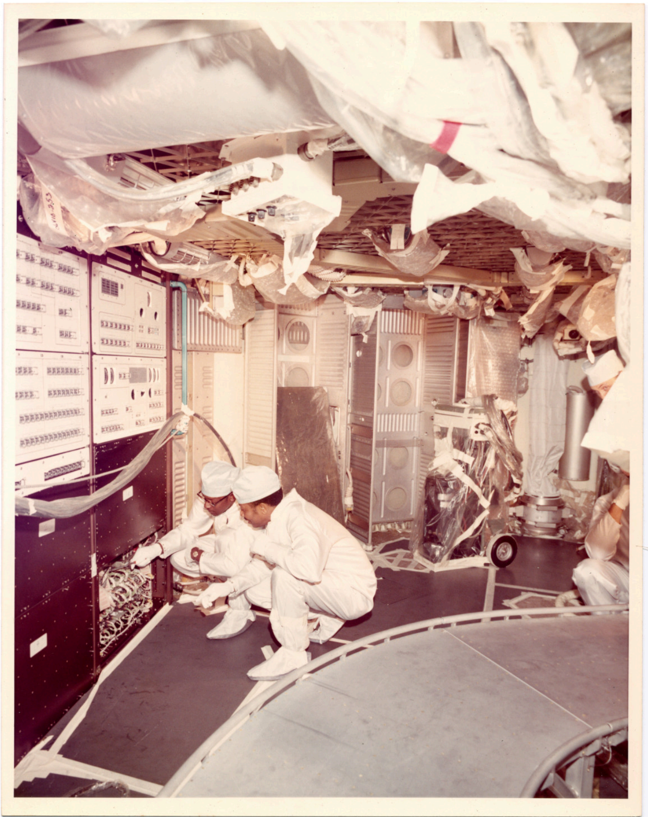
There is a still caption on the back which reads: "INSPECTING POWER DISTRIBUTION AND DISPLAY CONSOLE. OF OWS NO. 1."
