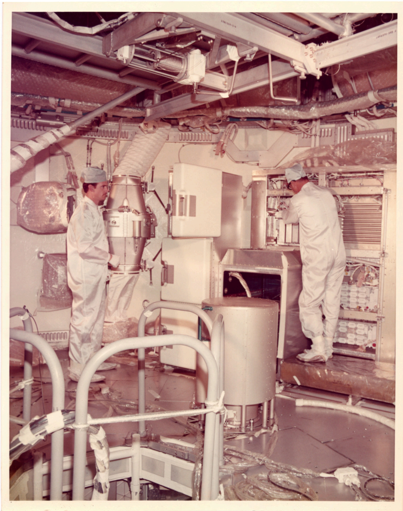
There is a still caption on the back which reads: "FAN CLUSTER, FOOD FREEZER AND REFRIGERATION SUBSYSTEM IN UPPER LEVEL OF OWS NO. 11"
