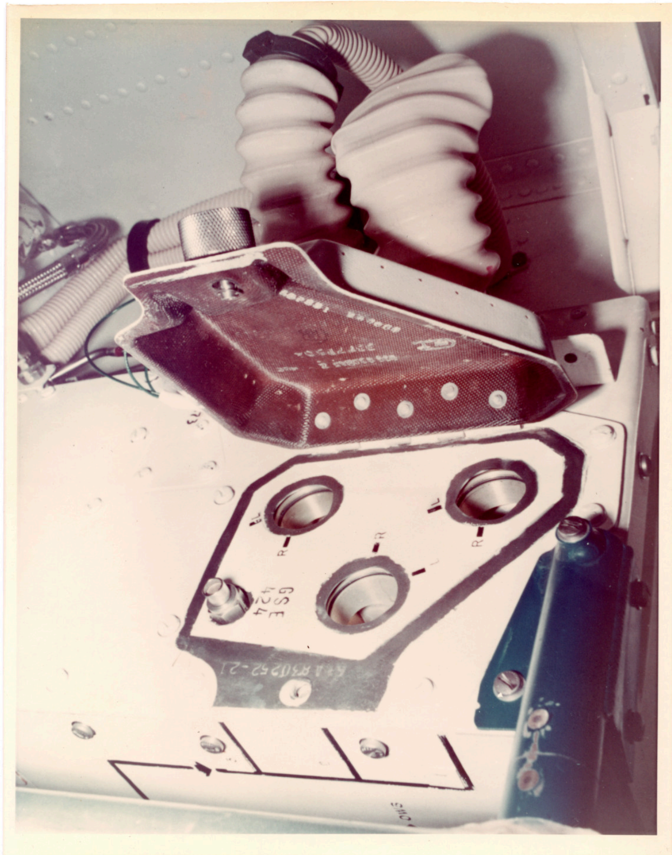
There is a still caption on the back which reads: "Airlock zone 1 closeup of O2 sensors location with sensor cover open and O2 sensors removed. MDAC Input for June."
