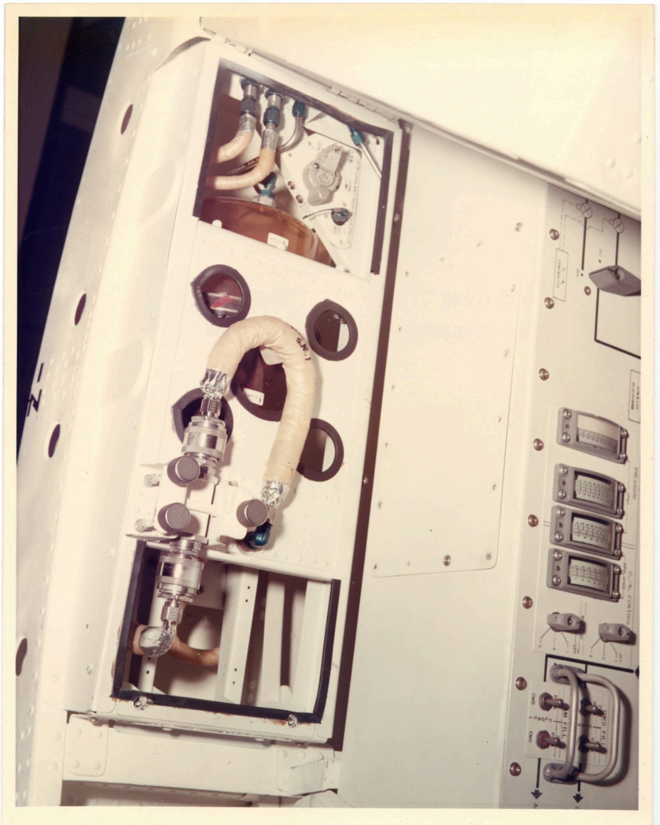
There is a still caption on the back which reads: "AIRLOCK NASA TRAINER IN MDAC-E BLDG-101 CLOSEUP OF ATM COOLANT RESERVOIR PRESS VALVE 235 (LEFT) AND ATM C&D H2O FILTER ASSEMBLY (RIGHT) NASA-1524"
