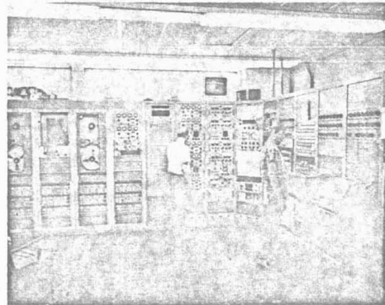
TELEMETRY GROUND STATION
