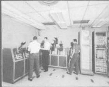
DATA ACQUISITION ROOM
