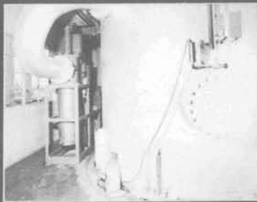
DUMP TANK AND VACUUM SYSTEM
