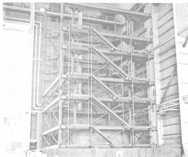
Figure III-4 - Construction Progress on the Hydrostatic Test Tower in the Vertical Assembly Building at Michoud
