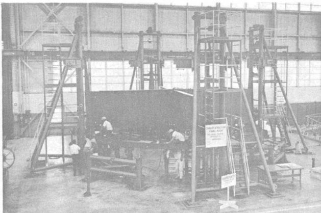
Figure III-8 - First Loading Operation of the No. 1 Thrust-Structure Final Assembly Fixture at Michoud. Lower Thrust Ring, Hold-Down Posts, and Center Engine Support Assemblies are seen Positioned in Fixture
