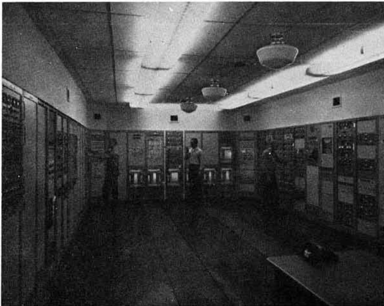
CONTROL ROOM, PERFORMANCE TEST CONTROL
