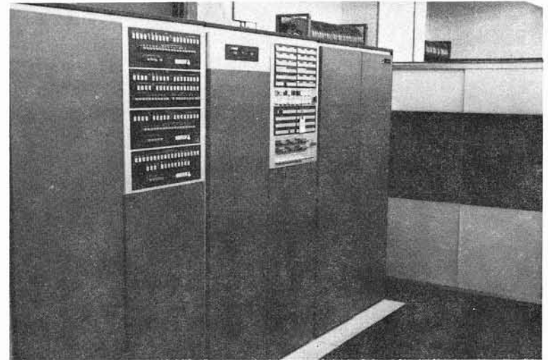
MSFC DATA CENTER 7740 COMMUNICATION SYSTEM
