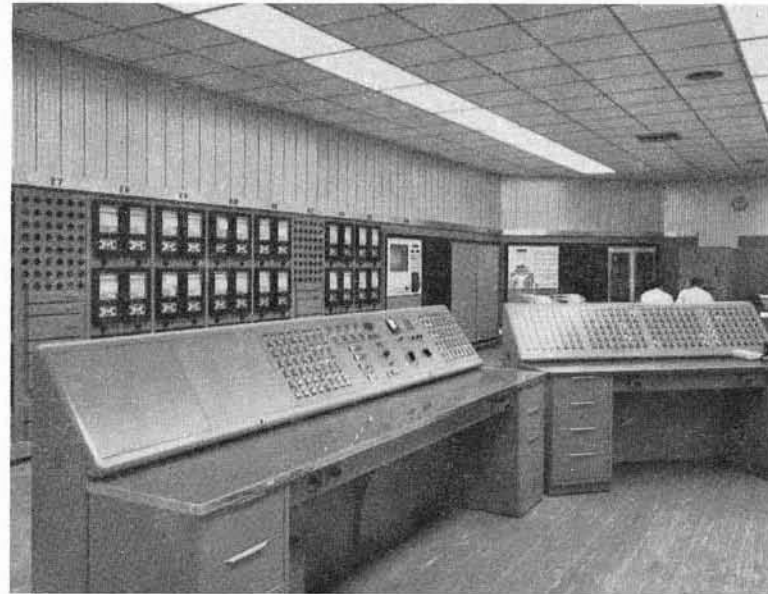
WEST BLOCK HOUSE RECORDER ROOM
