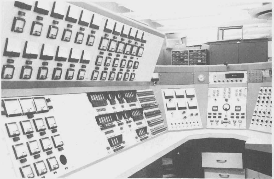
Control Console for 8000-kW Plasma Facility
