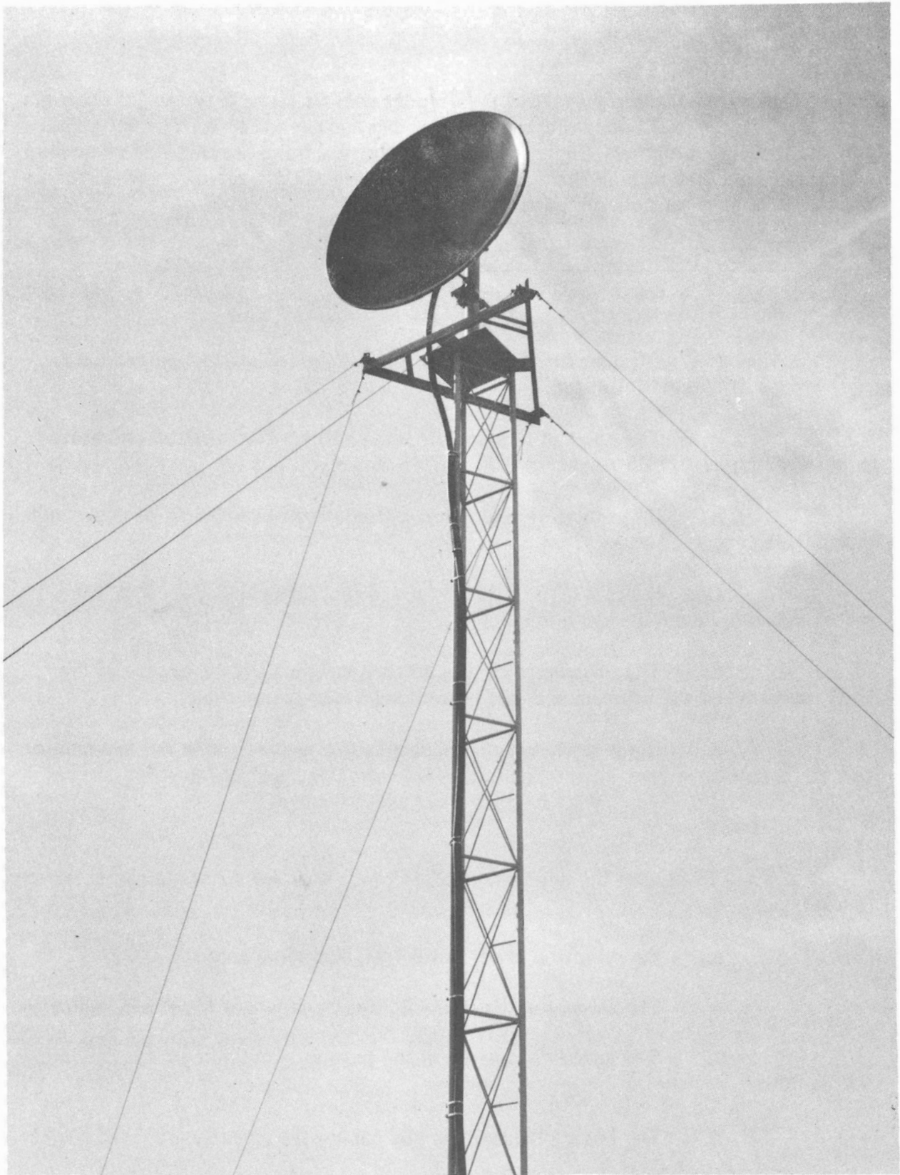
Figure B-2. Directional UHF Receiving Antenna and Tower
