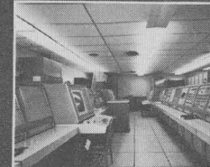
LCC CONTROL CONSOLES
