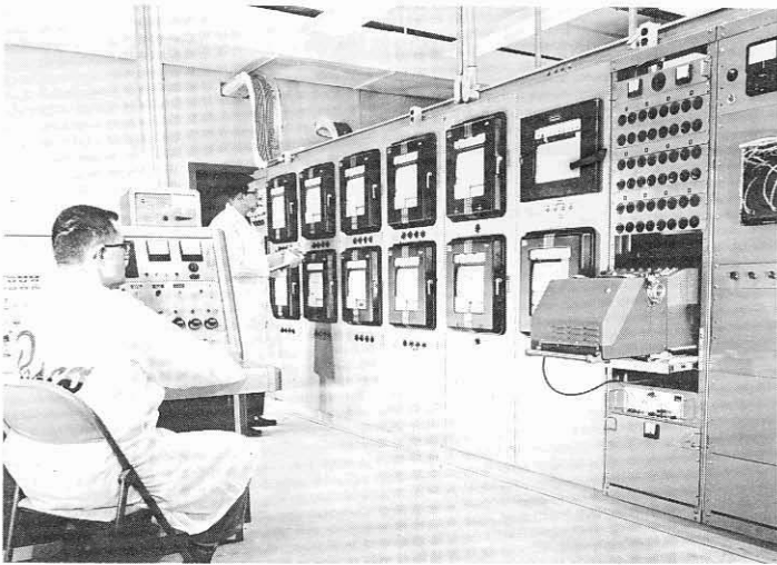
Central instrumentation and control for all test buildings at Pesco's Cryogenic Laboratory at Perry, Ohio. Control console with test monitoring instruments at left; recorders, center; oscillograph, calibrating controls and program boards at right.
