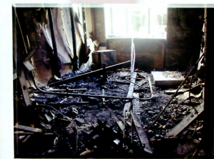
A burned office with original windows blown out. Fire spread easily through unrenovated areas without preventive sprinkler system.
