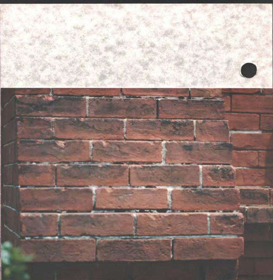
ERODED JTS. EDI TOWER
