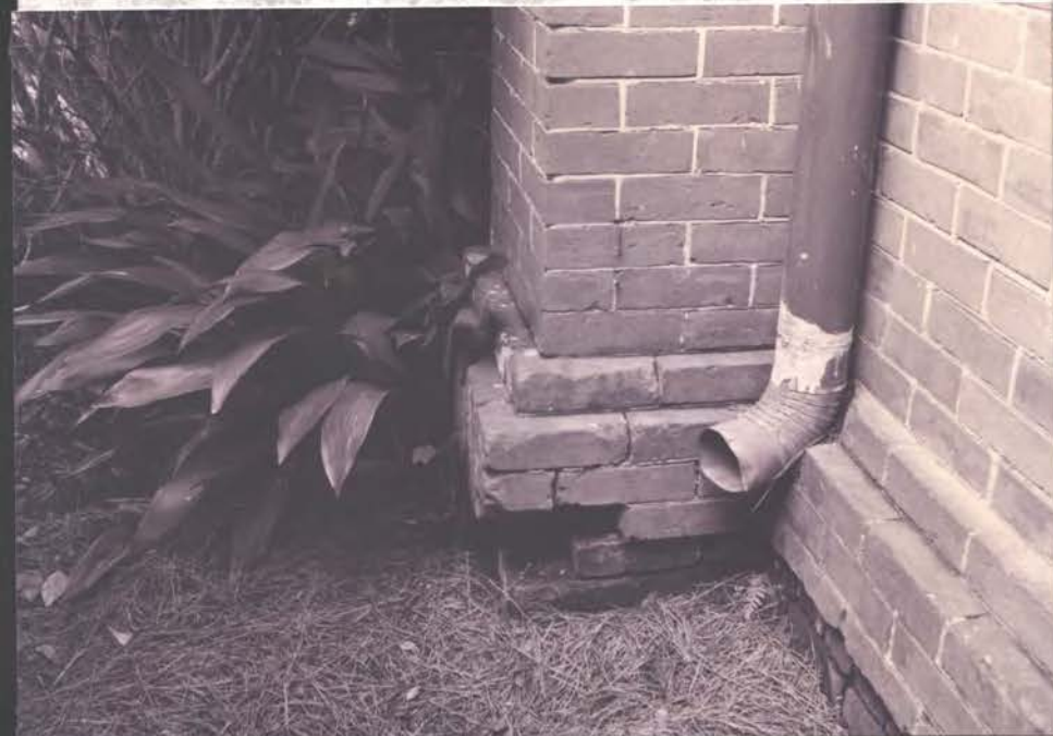
← D.S. DISCHARGE HAS ERODED JTS. (SHOULD DISCHARGE AT SOIL LINE)
