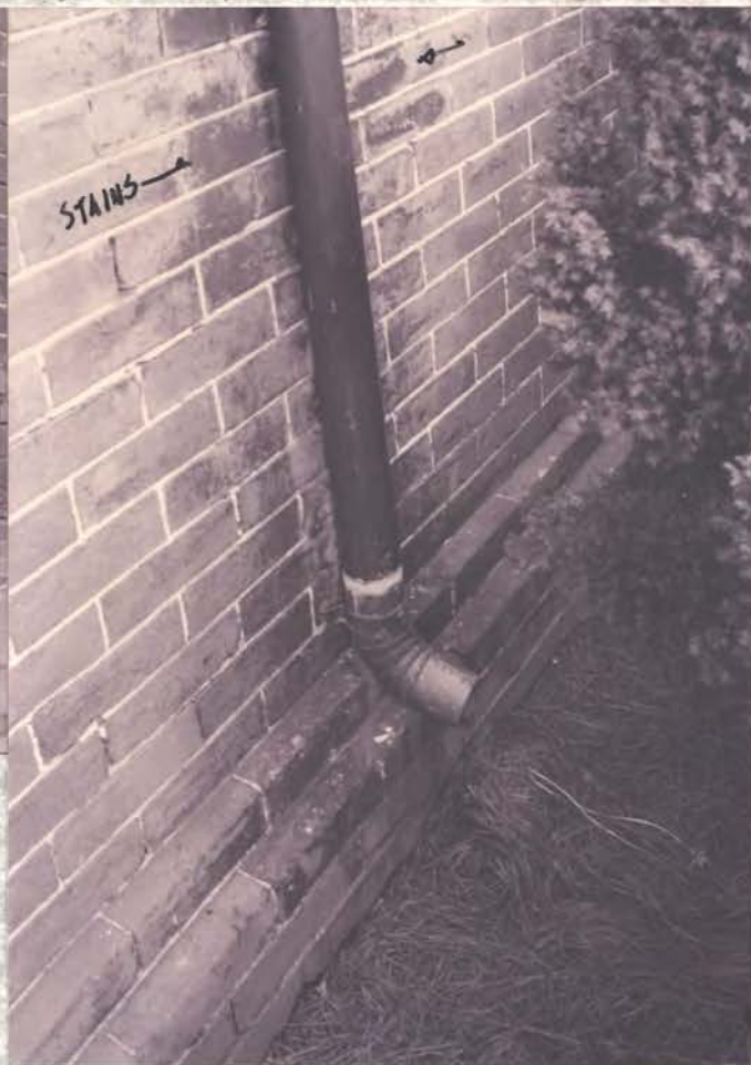
← STAINS ← NO WASHING OF STAIN INDICATES BLOCKED D.S.
