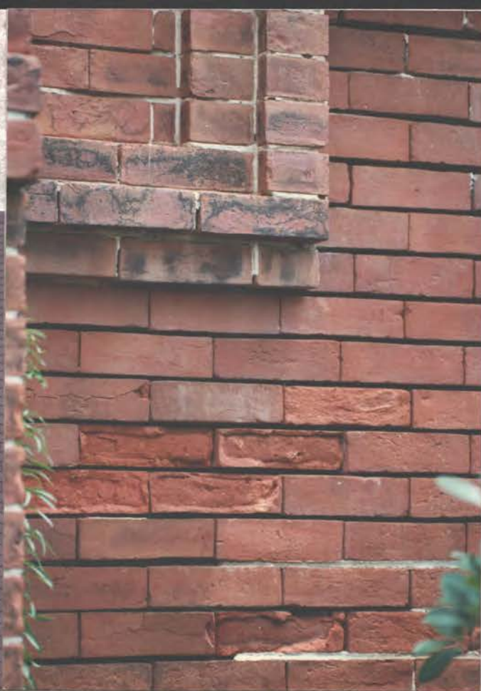
S. SIDE AT TOWER ERODED BRICK FACES + ERODED MORTAR JOINTS
