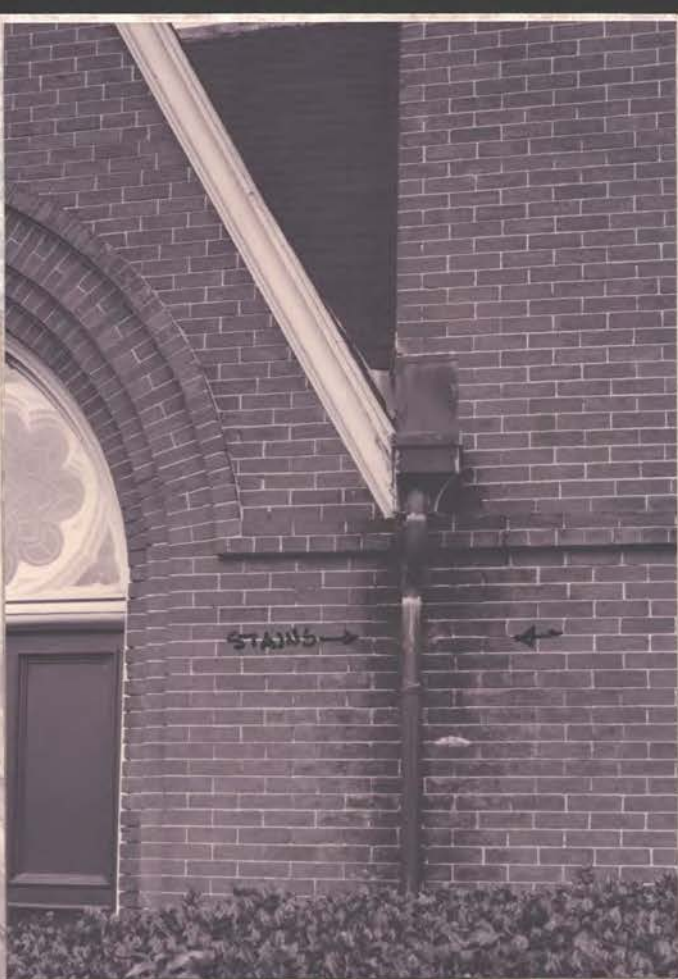
← STAINS INDICATE BLOCKED D.S. & WATER FLOW DOWN WALL (S. OF N.W. ENTRY) ←
