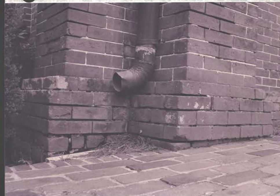
← DOWNSPOUT DISCHARGE 10" UP ON BRICK HAS ERODED JTS. - N. OF N.W. ENTRY (SHOULD DISCHARGE AT WALK LEVEL)
