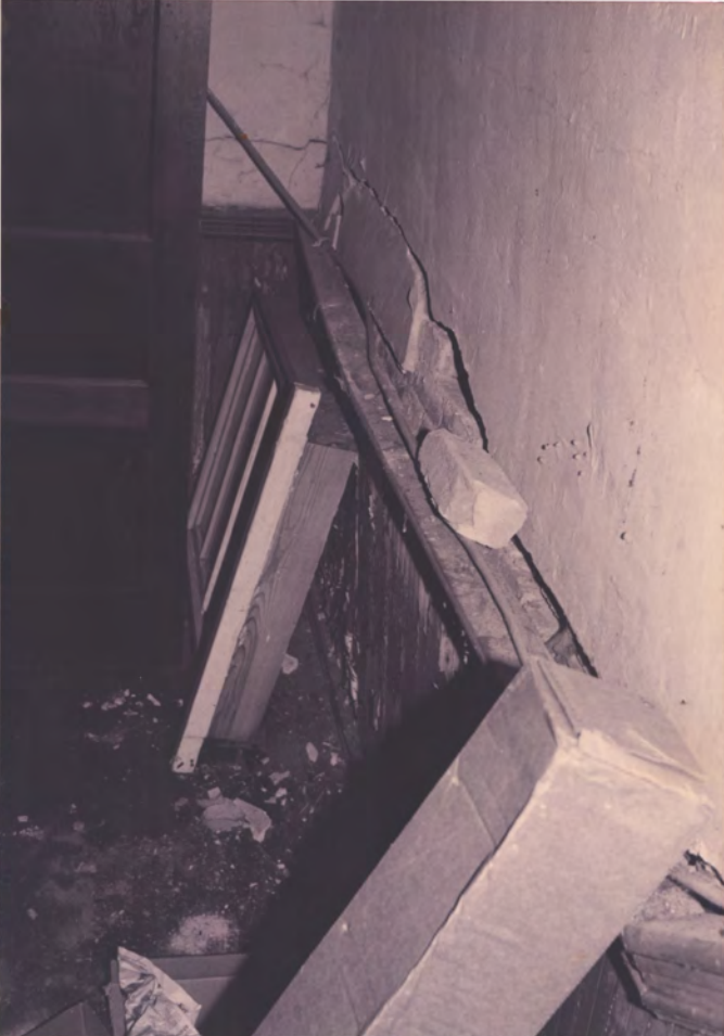
CHANNEL REAR WALL bowed out \pm 2"
