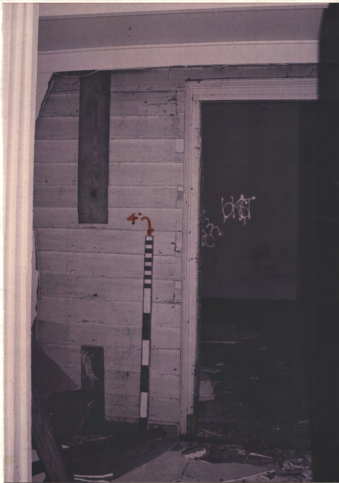
④ S.W. end of enclosed S. vic. porch (was ext wall) pW
