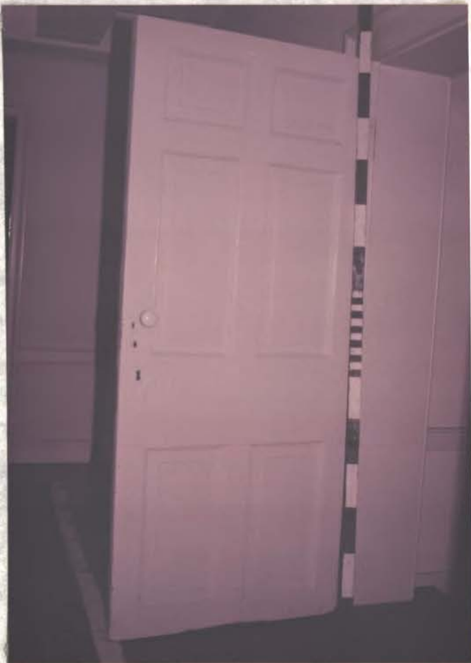
FED. G-P DOOR FROM FL. 1 N.W. SERV. RM TO REAR (W.) HALL
