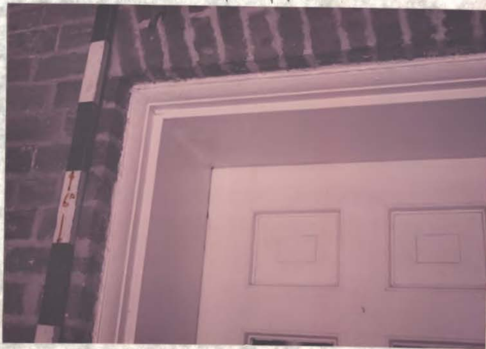
HEAVY REPOINTED BRICK (Sandblasted, portland cem., wide sloppy jts)
