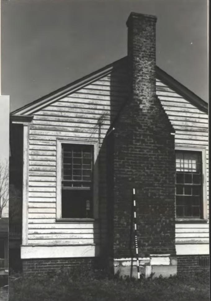
SOUTH WALL All looks 1850's except solid brick fndn. w/ full wall
