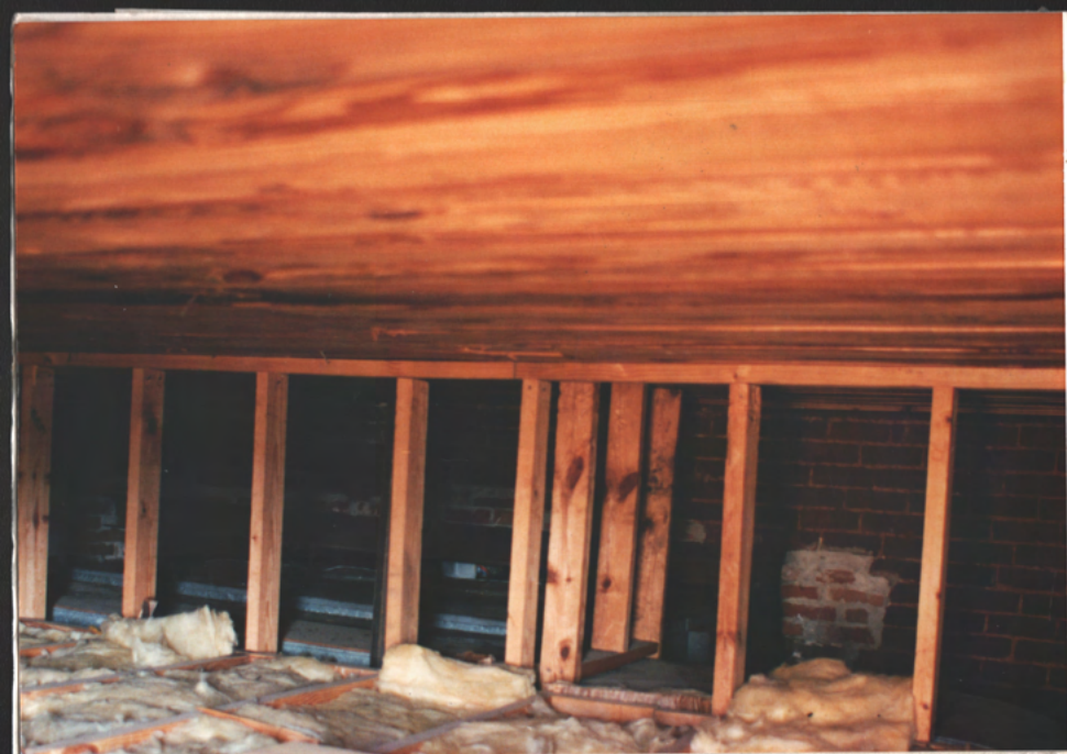
Pent. now empty except for return ducts seen. Once house AC equip (Equip - now in gabled attic)
