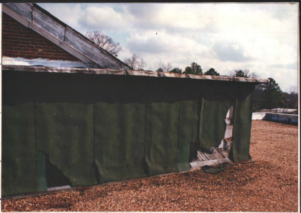
No * Door no more flash - water blows in. NEED FLASH
