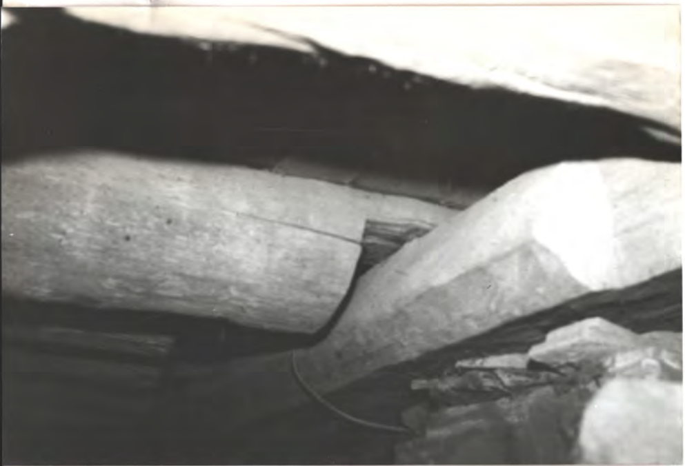
Purbeck J. joints under J. 1 of N.E. Rm, look SSW
