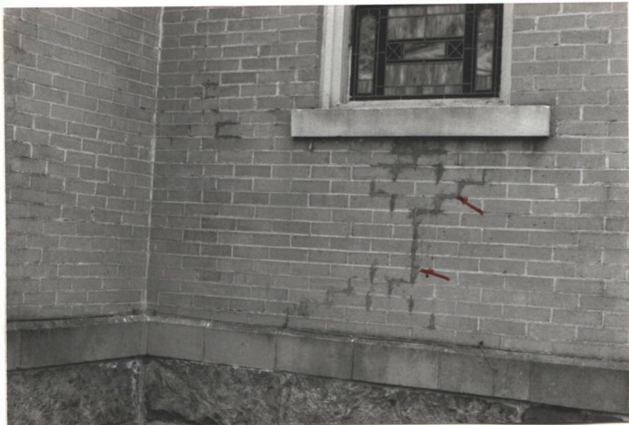
N. WALL AT VEST. AREA - DARK GRAY CEM. PATCHES
