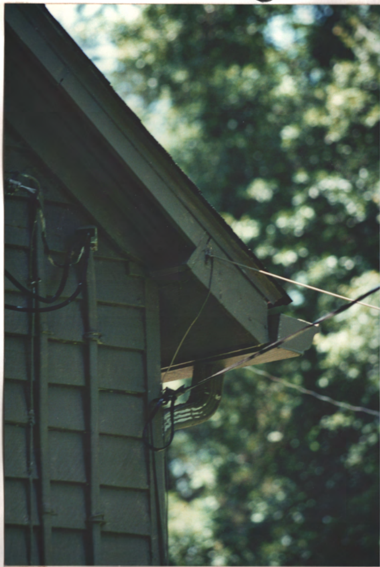
→ N N.E. Corner of E. Wing (Vic.?) Note joint in fascia indicating that the drip-edge was attached later
