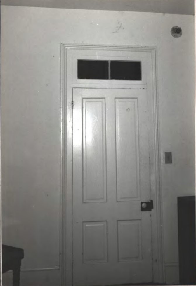
1870's rms. just N. of entry hall, looking S. (door opens into entry hall)
