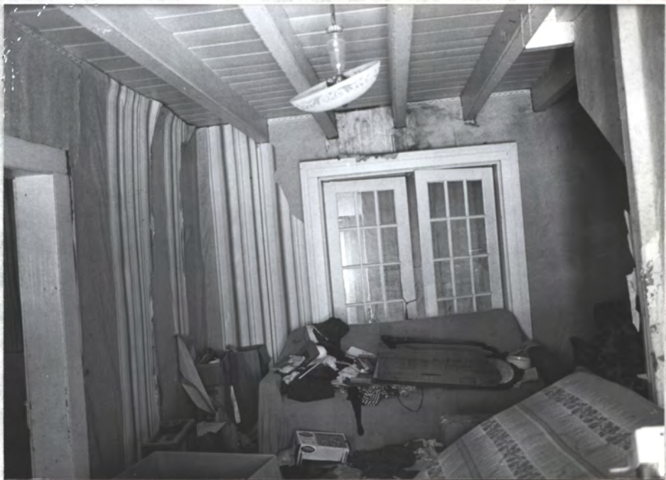
Entry Hall → N Rear door = 20th c. Banded joists of exposit - br. cel = orig. Stair ↑ up
