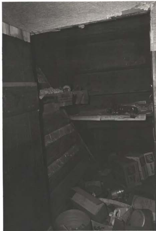
CLOSET SHOWING RISERS IN CLOSER DETAIL AND STORAGE SHELVES
