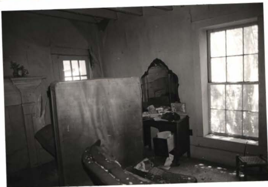
NORTH EAST VIEW OF ROOM 73. DOOR AT CENTER LEFT OPENS ON TO PORCH.
