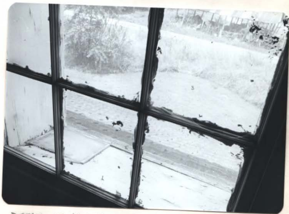
DETAIL OF ABOVE WINDOW SHOWING DEPTH OF WINDOW SILL CUT THROUGH LOGS
