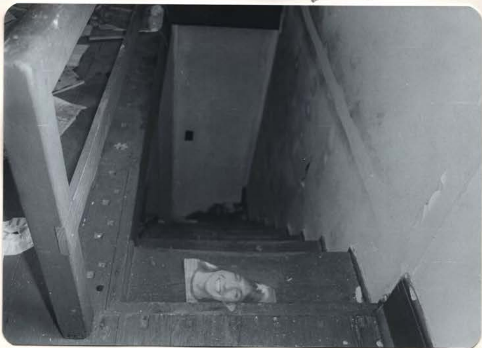
VIEW LOOKING DOWN STAIR IN ROOM B. NOTE HOLES WHERE EARLIER STAIR RAILING WAS PLACED AND ODD PATTERN OF HOLES. ALSO NOTE FILLED IN HOLES AT BOTTOM OF PHOTO.
