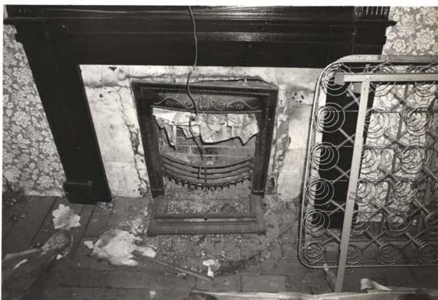
CLOSEUP OF FIREPLACE IN BEDROOM 3, MANTEL THOUGHT TO POST DATE ONES DOWNSTAIRS.
