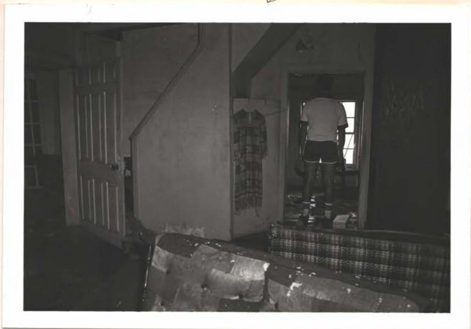
SOUTHWEST VIEW OF ROOM B. NOTE STAIRWAY IN CORNER AND DETAIL ON CLOSED BALUSTRADE, CLOSET UNDER STAIR IS IDENTICAL TO OTHER ONE
