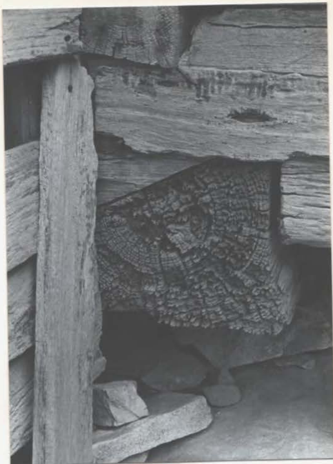
SAME NORTHWEST CORNER SHOWING STONE SUPPORTS OF LOGS AND JUNCTION OF 1ST ADDITION WALL
