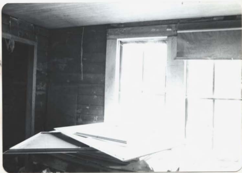
SOUTH WEST CORNER OF ROOM C SHOWING DOUBLE WINDOWS IN WEST WALL
