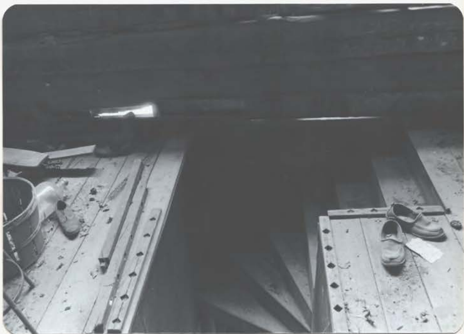
CLOSEUP OF STAIR OPENING - NOTE ↑ SUPPORTS FOR RAILING AND SINGLE RAIL AT LEFT
