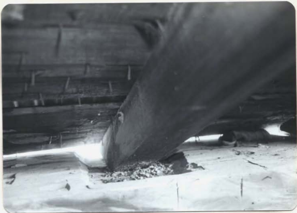
VIEW OF POCKET CUT FOR RAFTERS NOTE THAT BEAM IS SMALLER THAN POCKET CUT FOR ORIGINAL
