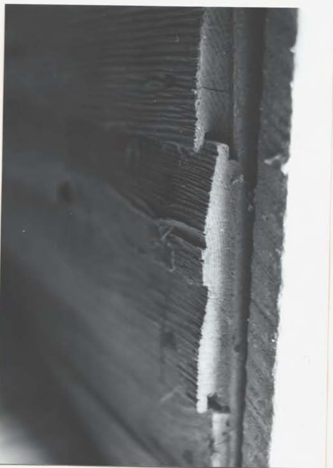
SIDING ON NORTH INTERIOR WALL - APPEARS TO BE AN EXTERIOR CLAPBOARD TAKEN FROM ELSEWHERE
