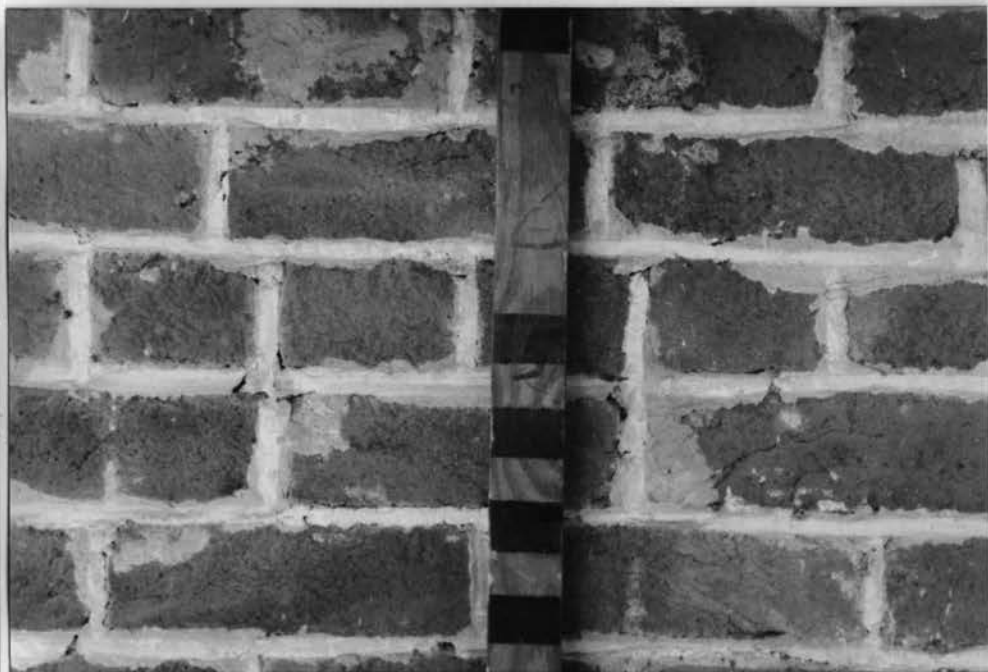
Note white paint "penciling" to emphasize brick jts. = typical of 19th c. (at Ekst Veranda)
