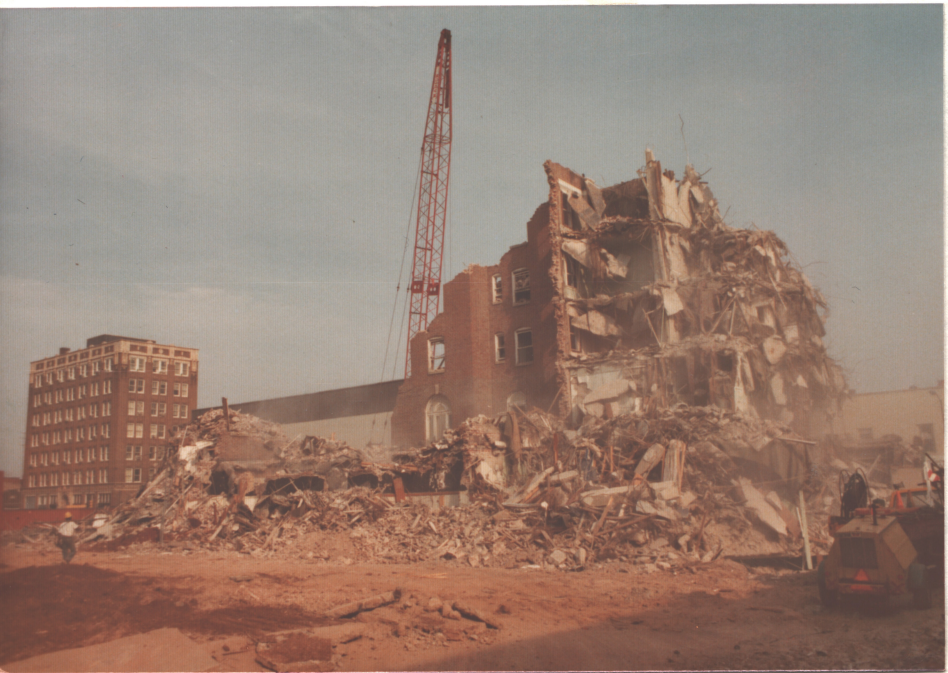
1975 photos — Twickenham 12th, 1914 ±, demol. Ralph Allen of Jones & Herrin, Arch. Demol. of N. half of block N. of Square for Parking Deck, J&H Arch W&H
