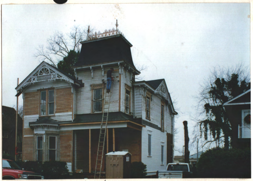
→ H E. F. FROM ↑ Joe Watson, owner of bldg. Porch being restored per two early photos of Somborn maps of 1894-98
