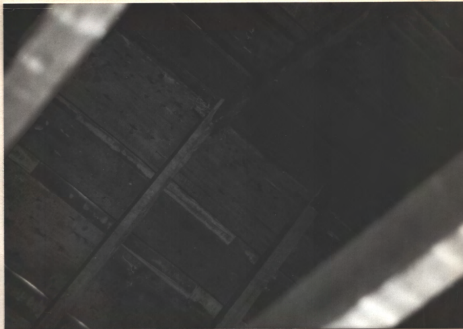
LAP + PEG CONNECTION AT ROOF RIDGE VERY WIDE ROOF-DECK SLAB PLANKS FOR WOOD SHINGLES = TYPICAL FED.
