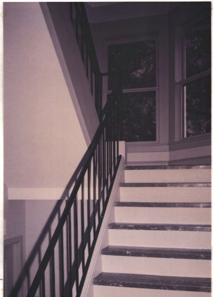
1996 rem. Fire - stair
