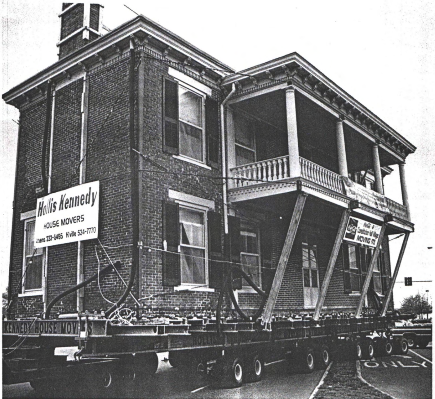
The large number of wheels and the hydraulics allowed crossing curbs, sidewalks and traveling the one mile of highway without damage. Six of the eight dollies are in caster mode.
