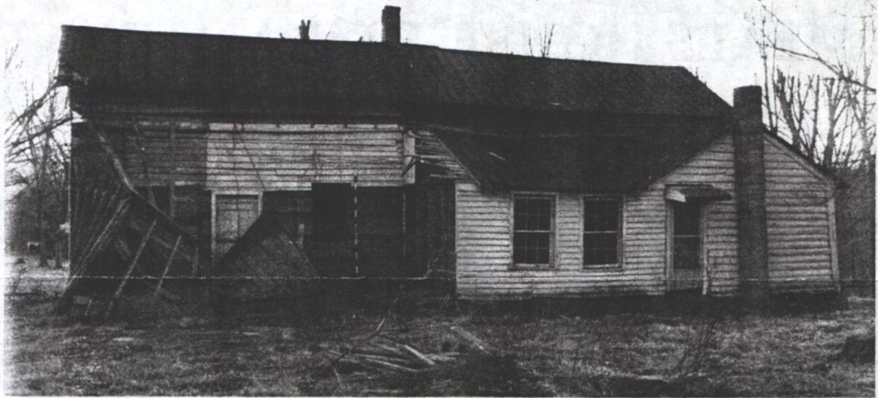
Rear view, February, 1993. The earliest addition, ca. 1860, has fallen down at left. Photograph by Harvie Jones, architect.
