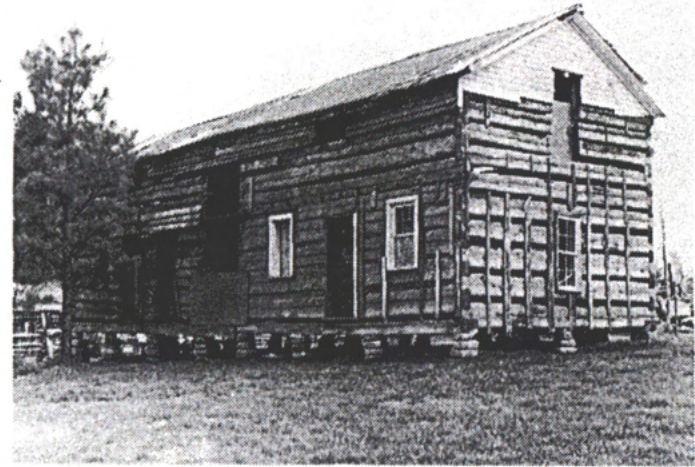
Above: James A. Meals house on site at Burritt Museum. The clapboard siding has been removed to determine which logs need to be replaced. 1994.
