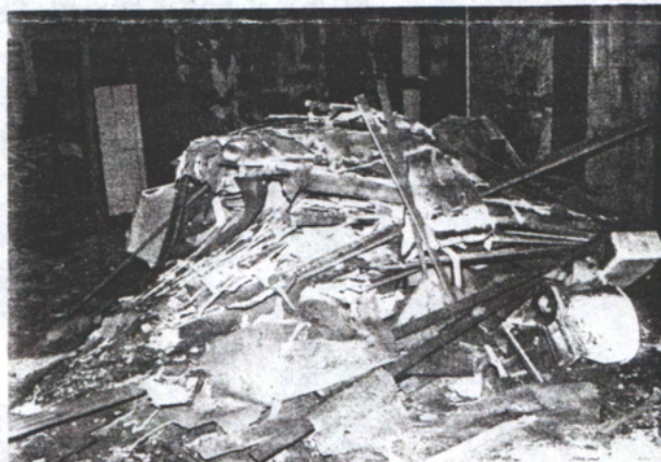
Restoration under way in the west pen, January, 1994. All post-1850 elements were removed. Photograph by the author.
