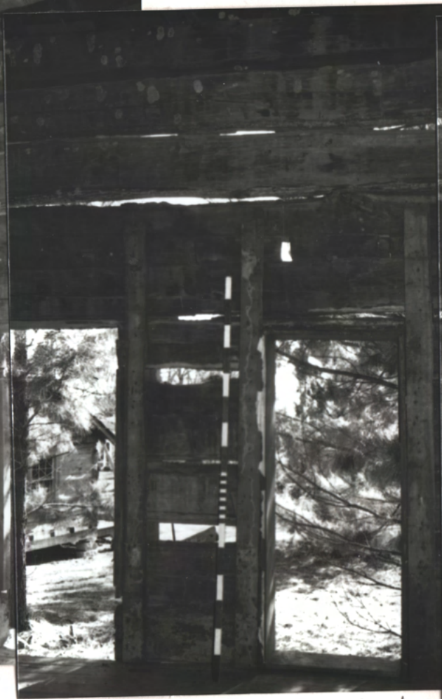
Orig. opry. w/ later rotting same frame
