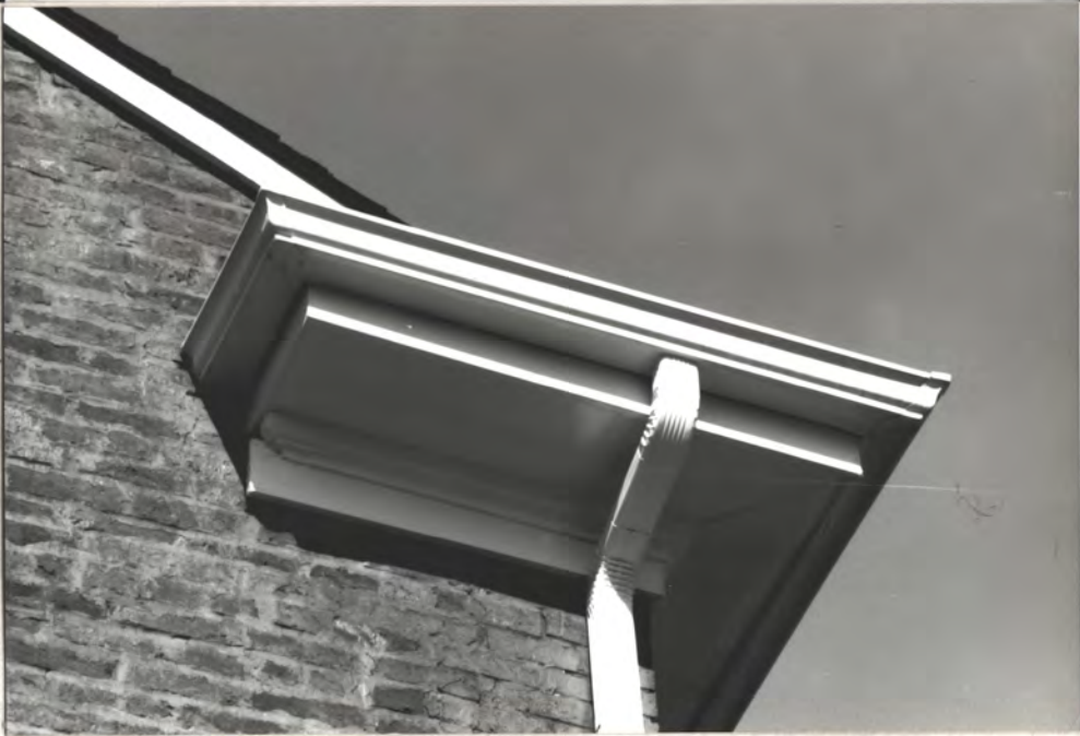
Main roof cornice. Gutter is modern & replaces a wood cornice (not by J&A)
