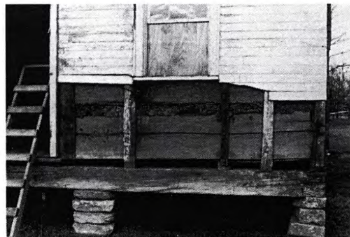
Below: Removal of 1900-era siding to determine condition of logs. During the restoration, the house will be resided to bring it to its 1850 appearance. Note the chinking and mud daubing between the logs. 1994.
