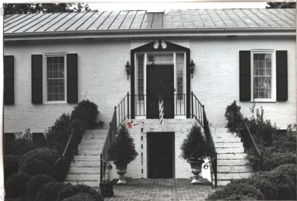
Steps of "pediment" at entry = ± 1940 & ± 1970 respectively. No record of orig. entry design.
