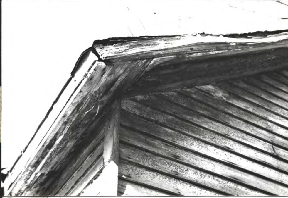
front S.W. corner. Typical Vic. roof detail (note pattern of soffit boards)
