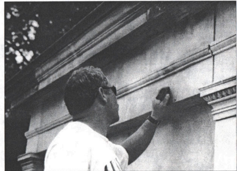
Detail of Mary Bibb Mausoleum, Maple Hill Cemetery, after restoration. A craftsman from Wasco, Nashville, finishes the restoration of the damaged stone. Courtesy Margaret Belle Crow.
