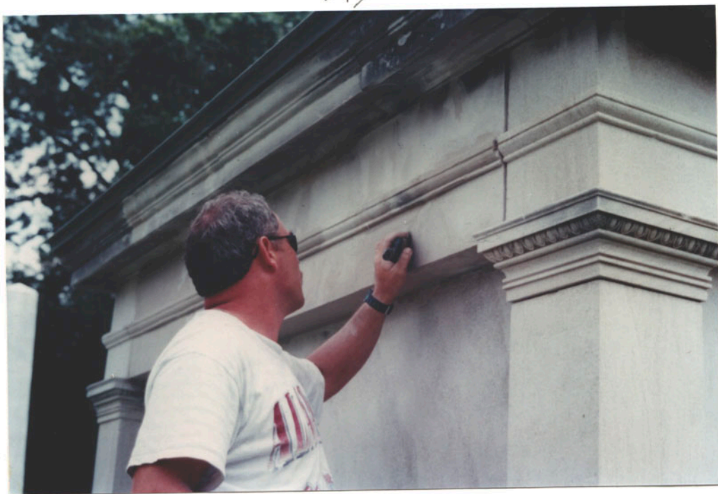
AFTER - resurfaced with "Jahn" restoration mortar by "WESCO" of Nashville. All arch. work donated by H. Jones
