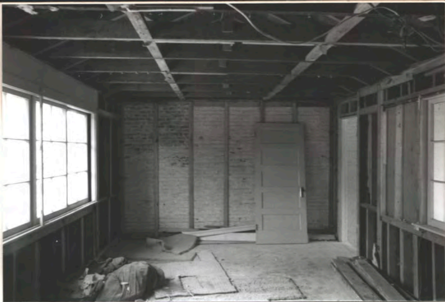
N ← "LINK" RM. - MOD. - CONNECTS MAIN HSE W/ SERV. WING AT 2ND FL.
