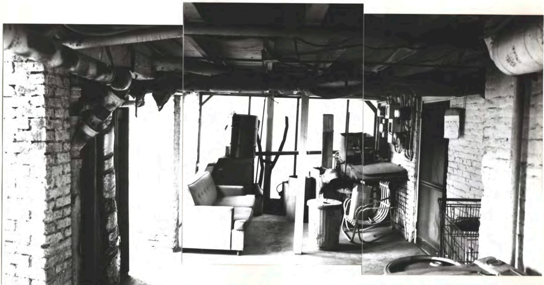
N.W. REAR PORCH AT GROUND LEVEL STRUCTURE IN FOREGROUND APPEARS TO BE FED. PORCH COLS. + JOISTS
