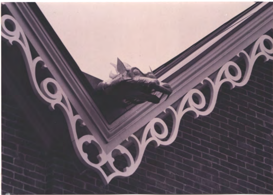
Copper cornice part at north valley made by Overthor Huber-Delke ( o "Copperworks" Co., Detroit)
