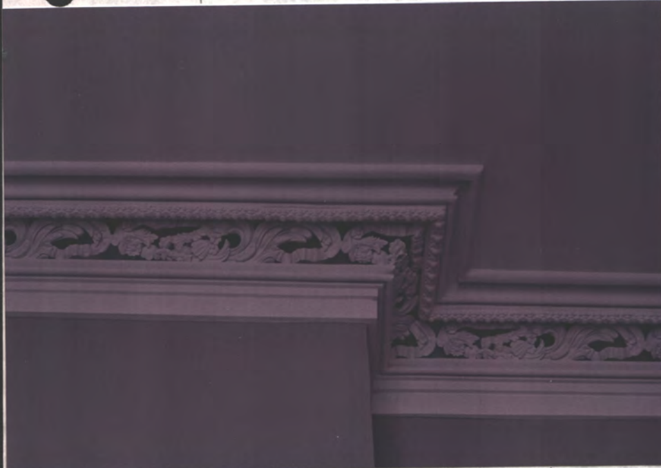
Restored hollow-plaster cornice. W. PARLOR Most destroyed or damaged by water in f after 1973 fire. Has sat for ± 2 yrs w/o a roof.
