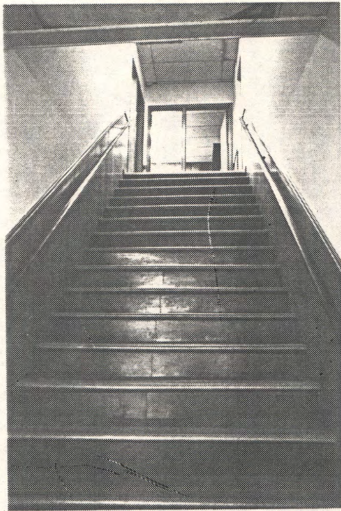
PHOTO 8 - 20TH CENTURY STAIR ON OPPOSITE SIDE OF BUILDING FROM ORIGINAL STAIR (PER CONTRACT AND EARLY PHOTO).
