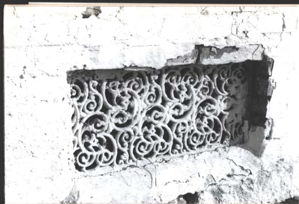
Added Vic. finish vent - front wall Originally were more at front, per brick evidence broken brick jambs N →
