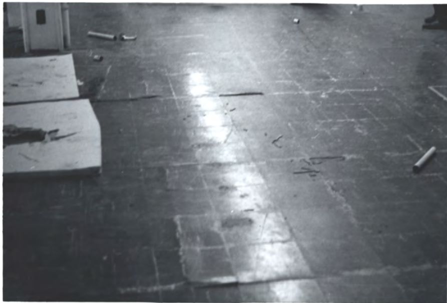
buckled 1960's asphalt tile fl. Lincoln Mills
