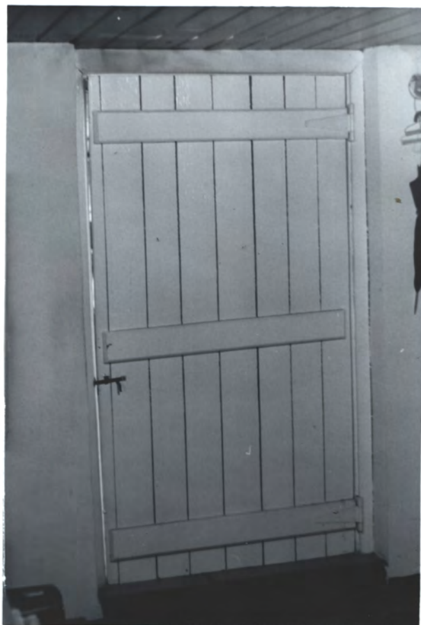
Grnd Fl. west door under N.W. (orig) part - door may be orig, except mod. hinges (?)
