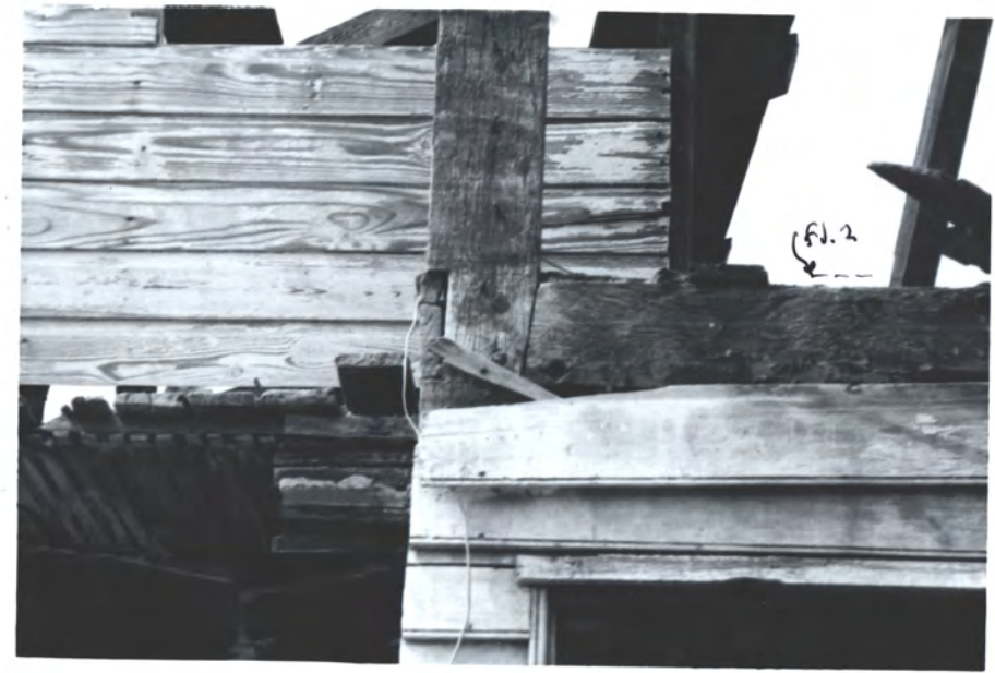
N. front beaded pre 1830 clap'd Mortise, tenon & peg jt. in fram. FGP. CLAP.
