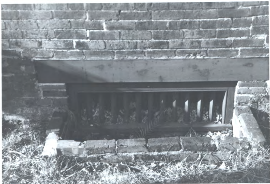
Typical Fed. Foundation vent. Brick "fence" is later, as ground built up
