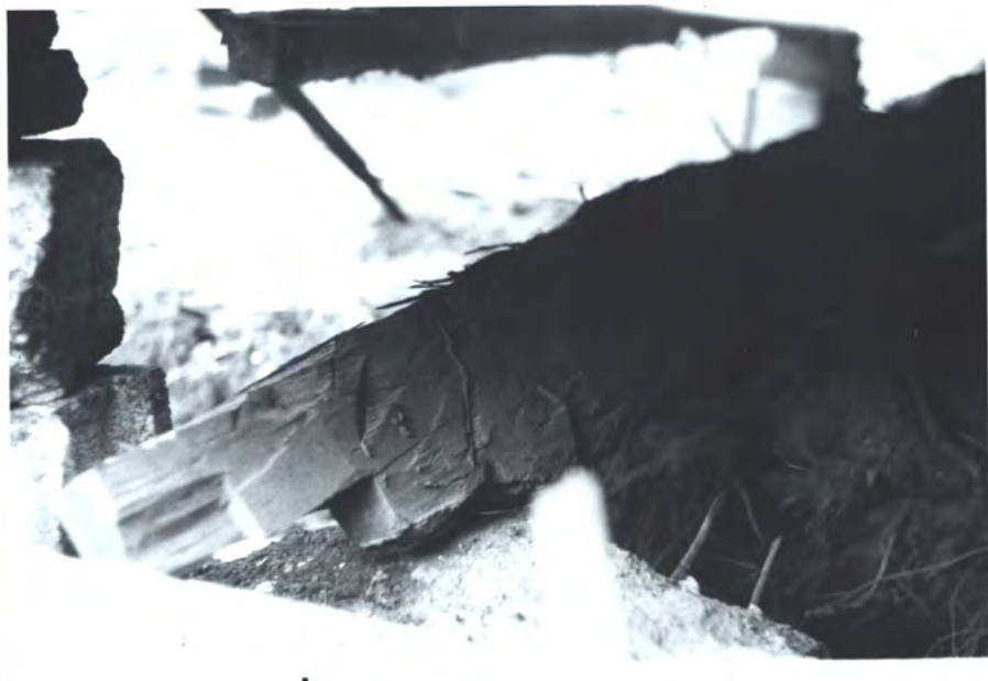
S.E. corner of beams (E.W.M) Hem. joist confirms S. beams is part of orig. Fed. period structure (part)
