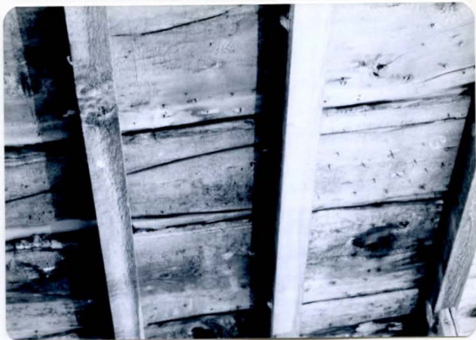
ATTIC - RAFTERS AND ROOF SHEATHING - ALL OF CEDAR AND WITH ORIGINAL CUT ROOFING NAILS PROTRUDING
