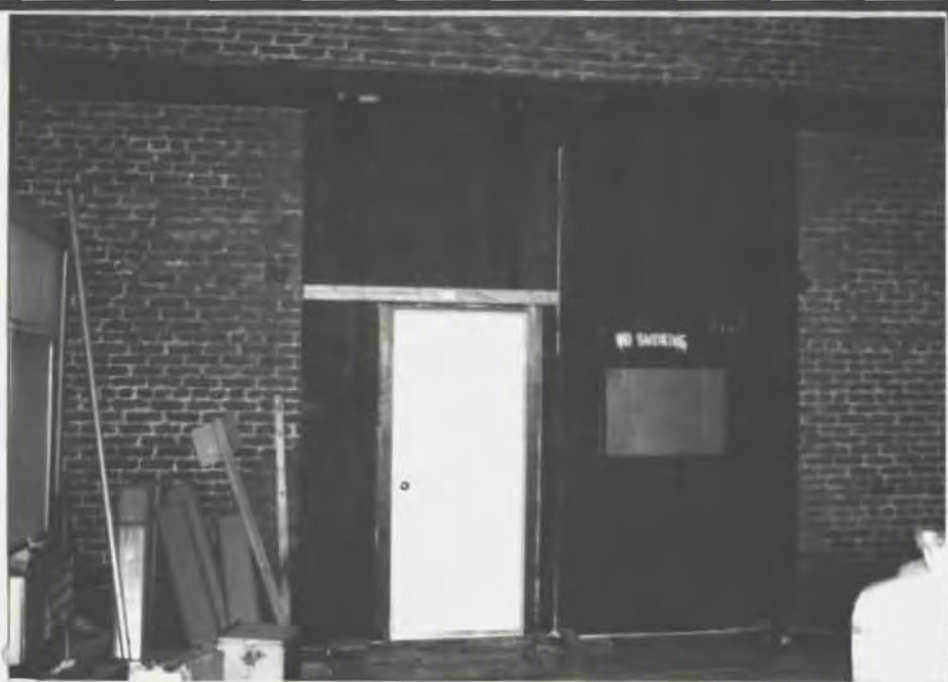
No. Door w/ 1980's door chopped into it
