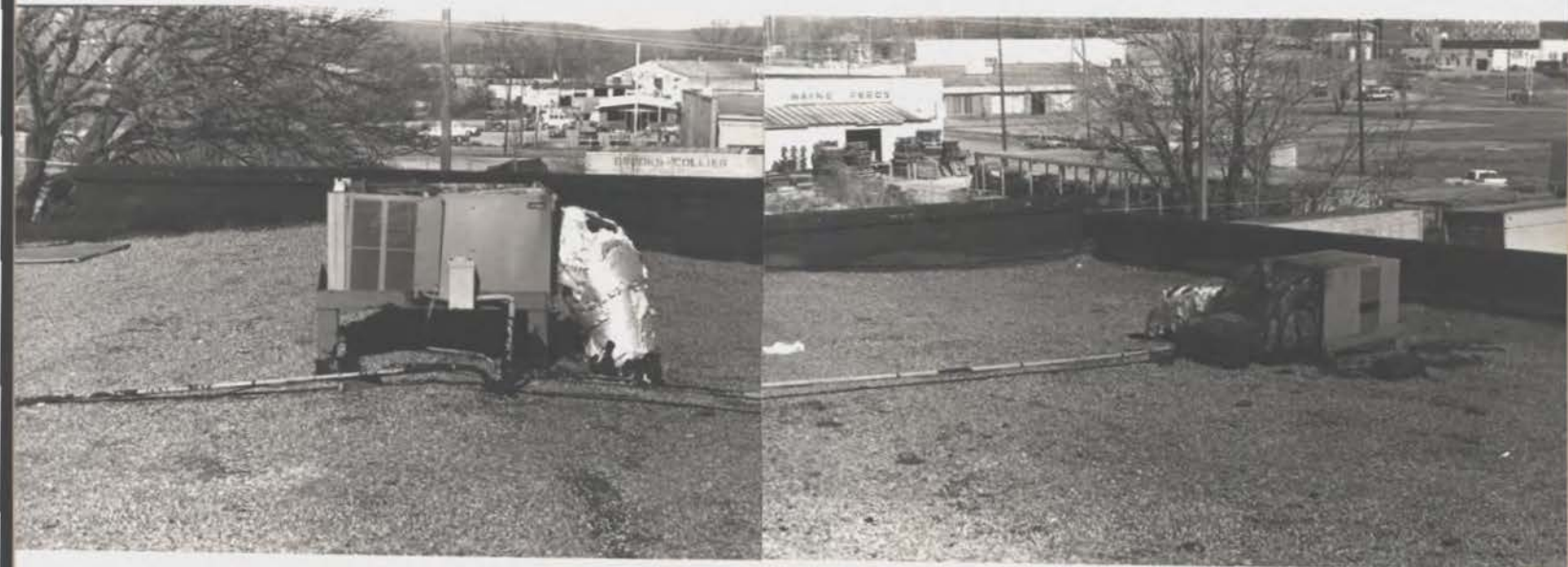
HVAC units on roof.
